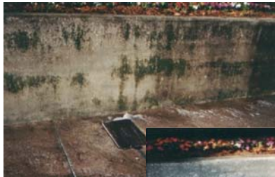
Before and After Photos of what Algae Mildew Cleaner can do!
