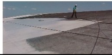
Roof Cleaning at Panther Stadium, Sunrise, Florida (The grey areas are mildewed The white areas have been cleaned)
